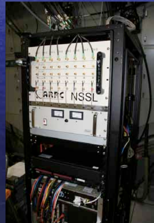
Installed rack w/ digital receivers
